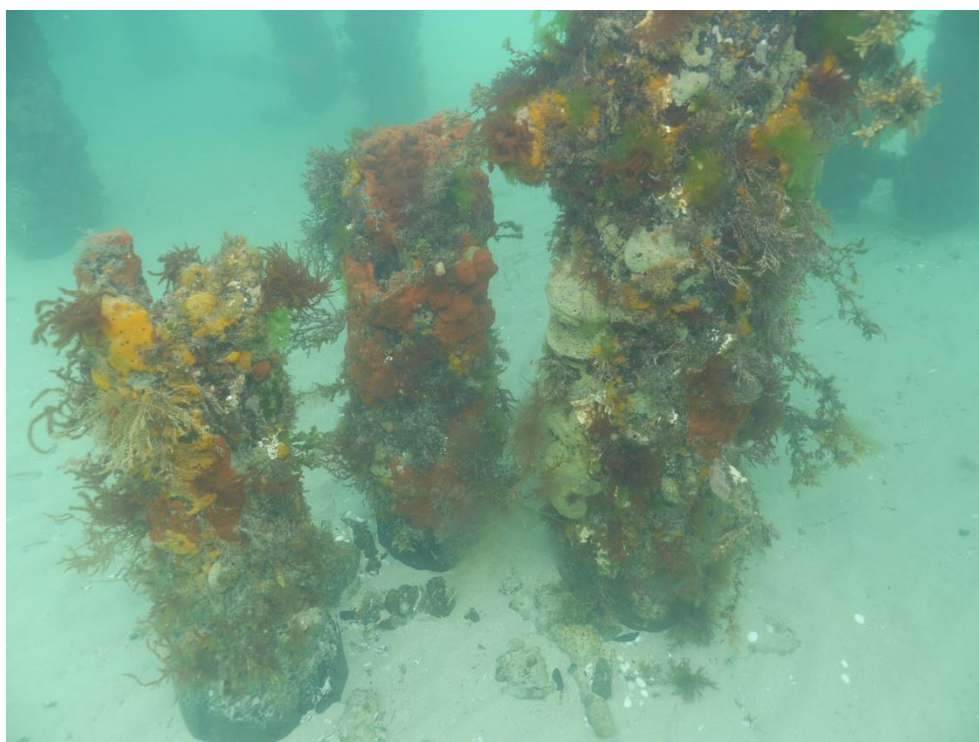
Figure 18 Marine life on existing cut-off piles at Rye Pier near lower landing, CEE September 2019
