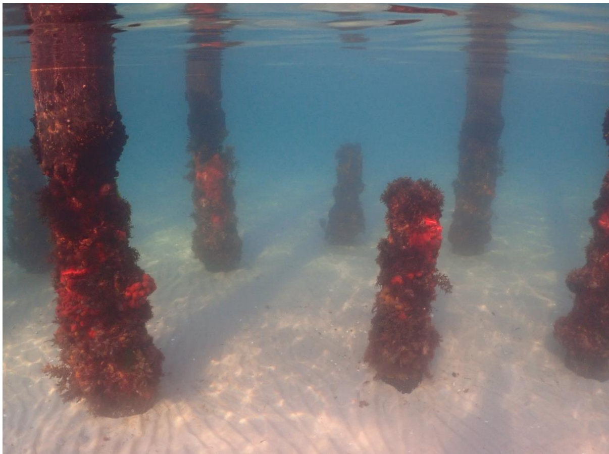
Figure 12. Piles at around chainage 140, Survey Water Depth 1.9 m, Depth to CD 1.0 m
