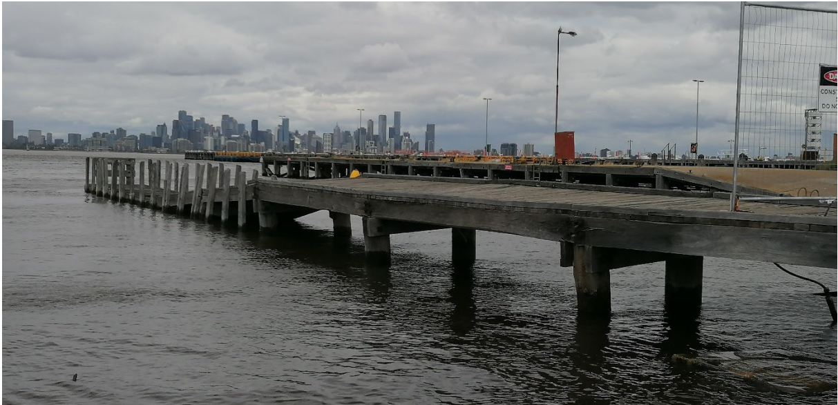
Figure 30. View of Commissioners Jetty from the west side, which is currently closed to all access due to poor condition.
