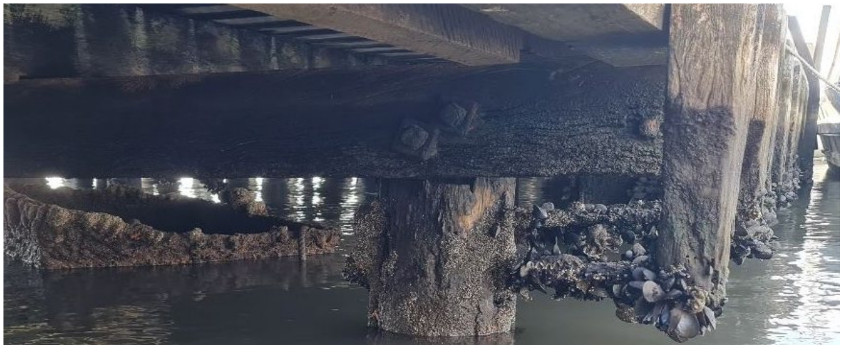
Figure 28. Timber elements below the low landing showing signs of deterioration. (Source: AWM 2022a)
