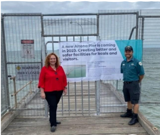
Image: The Minister for Ports and Freight celebrates commencement of Altona Pier replacement with Parks Victoria. February 2023.
